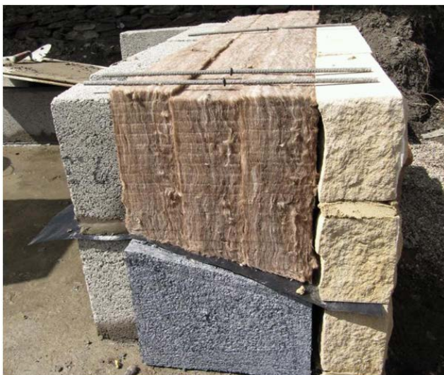
Figure 39 Fully filled 300mm cavity wall construction with sandstone facing (courtesy of Green Building Store).
