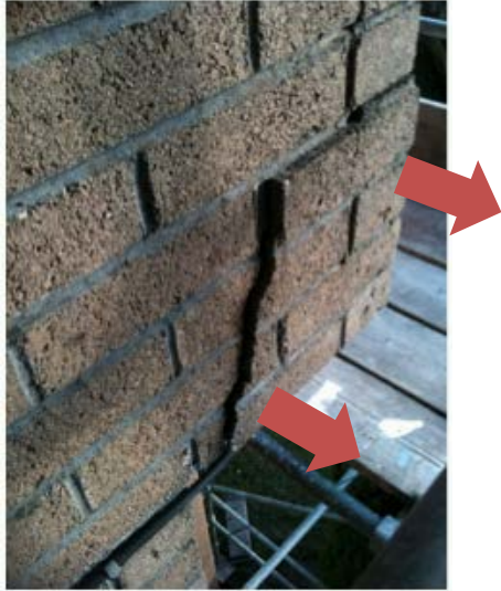
Figure 40 Ice expansion damage to the bottom of a poorly draining cavity wall (courtesy of J.Morehead)
