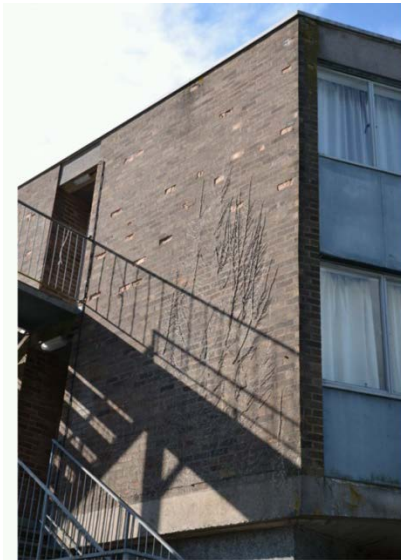
Figure 41 Spalling damage to a brick facade caused by driving rain and subsequent freezing
