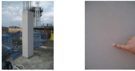
Figure 2.1: Surface finish for a column using SCC with no repairs or “rubbing down”
