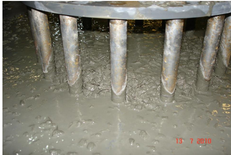
Figure 4.10: Fibres and large aggregates are nested around the steel rods in an earlier trial version of Mix 6 that had met the flow-ability criterion
