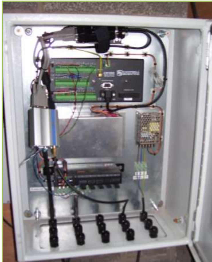
Figure 3.15 – Photograph of the installed data-logger and modem within the protective enclosure.
