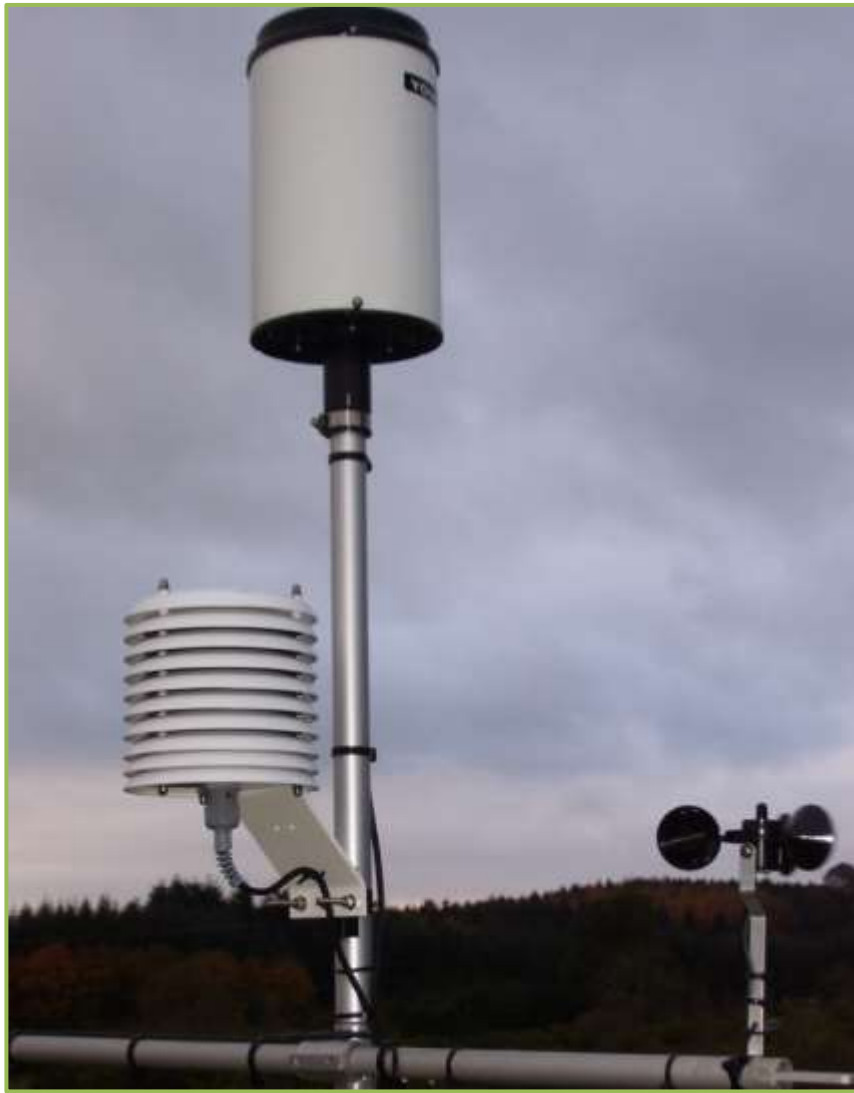
Figure 3.11 – Photograph of the installed anemometer along with the remaining climatic sensors.
