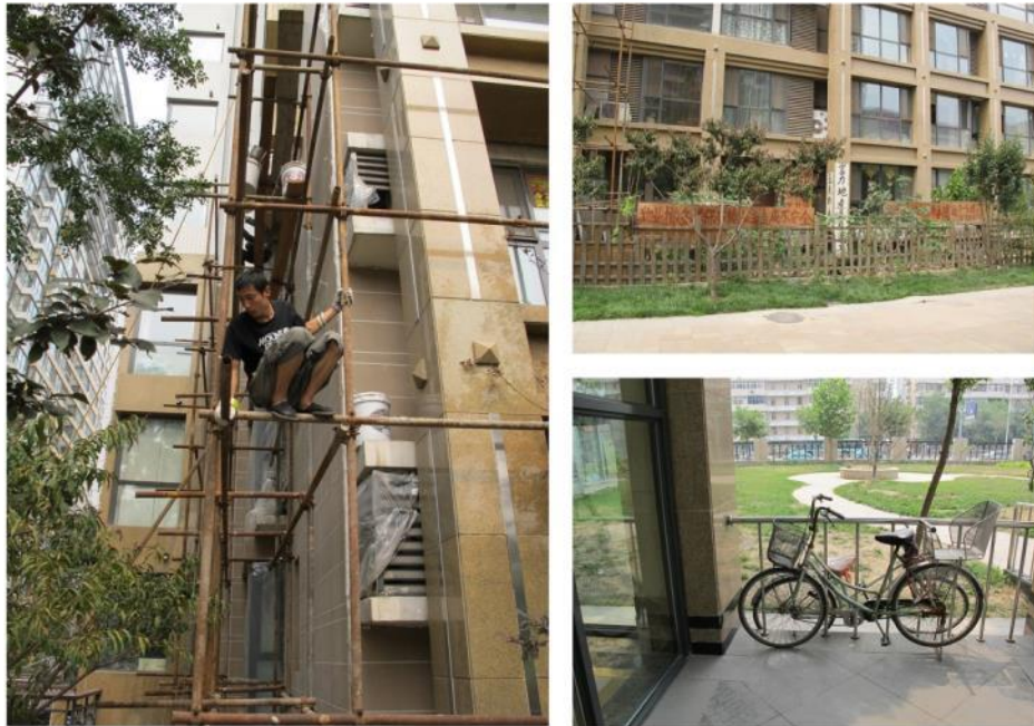
Figure 5- 48 Problems of Management and Maintenance of Case 3 Left: repairing the wall tiles; Right top: banners hung on the building to protest against the developer; Right bottom: the bike was locked on the railing of the entrance.
