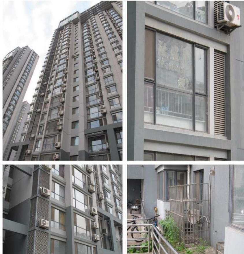
Figure 5- 62 Outdoor Units of Air Conditioners Fixing on the External Walls
