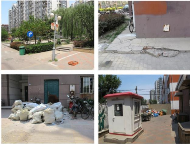
Figure 5- 15 Lack of Maintenance of Public Spaces and Facilities of case 1
