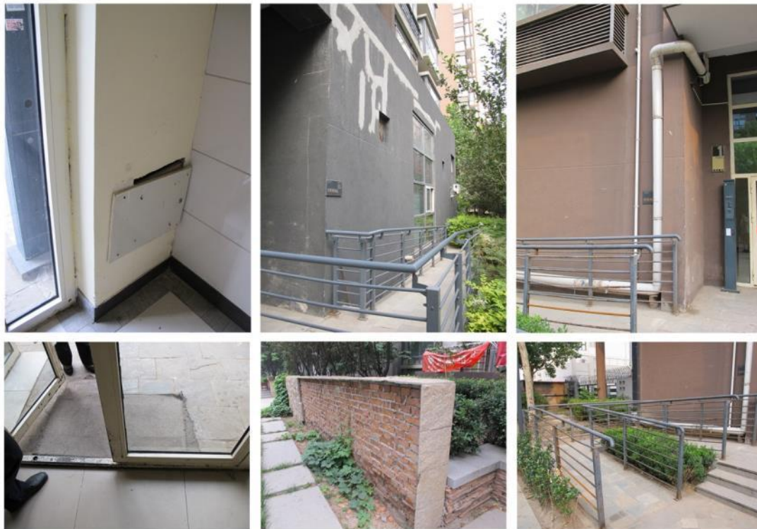
Figure 5-36 Problems of Construction Quality of Dwelling Buildings in Case 2
