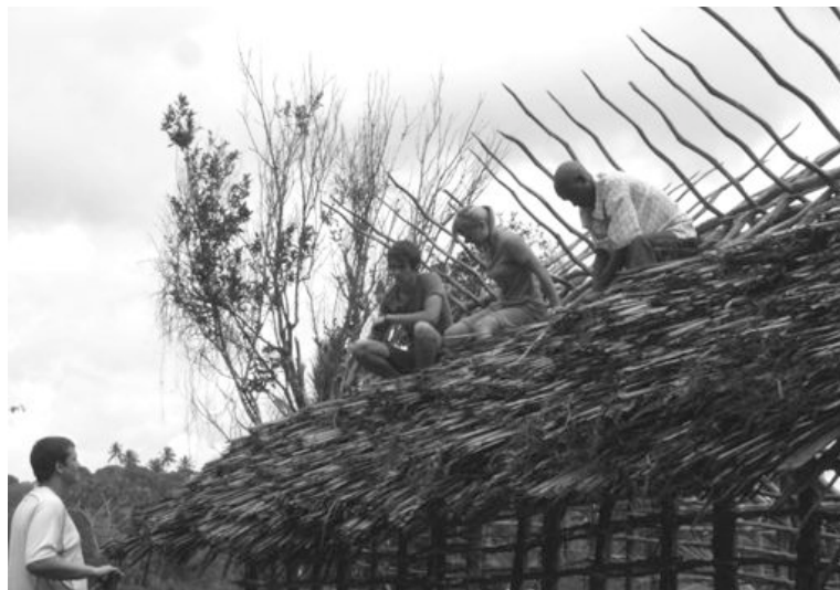
Figure 24. Volunteer tourists completing the roof on one of the Mama's houses. Source: Participant.
