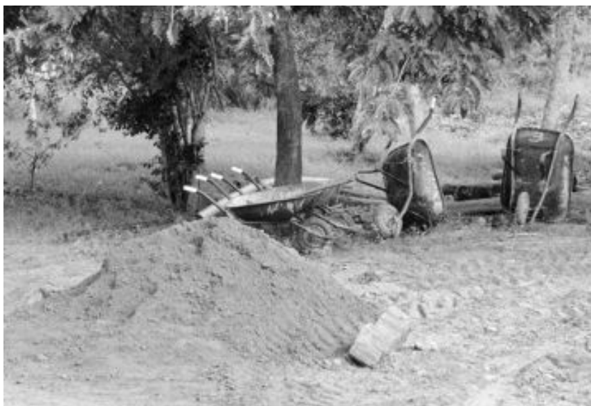
Figure 19. Imagining building work: construction site for one of the volunteer projects. Source: Author.
