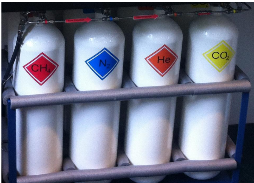
Fig. 3.28. Gas reservoirs including four pairs of diving cylinders (one standby and one in duty), secured inside a metal rack.
