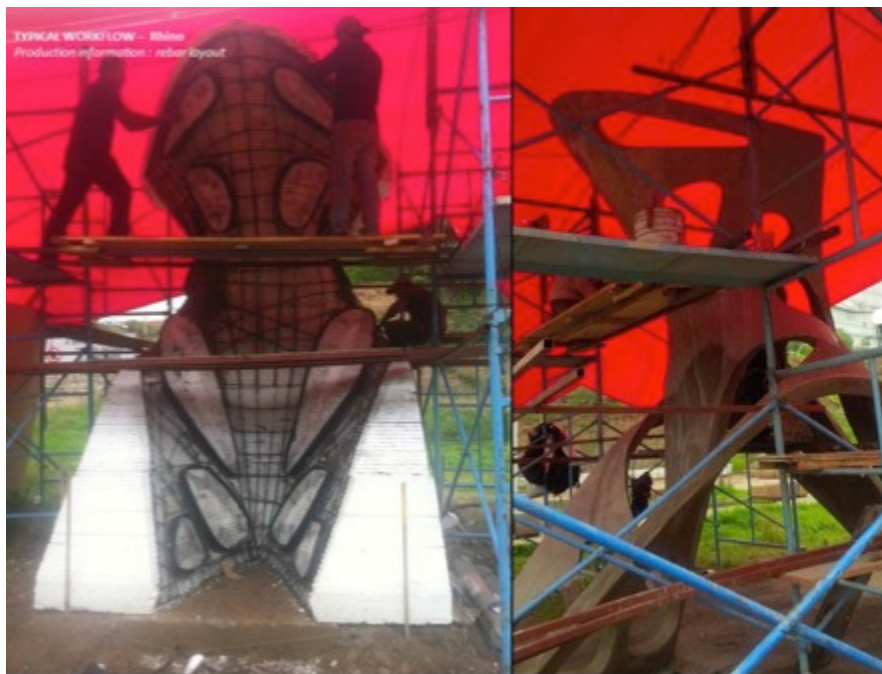
Figure 14: (left to right) Perimeter edges cover with reinforced wire plastic slip. Piece after concrete was poured and formwork removed.
