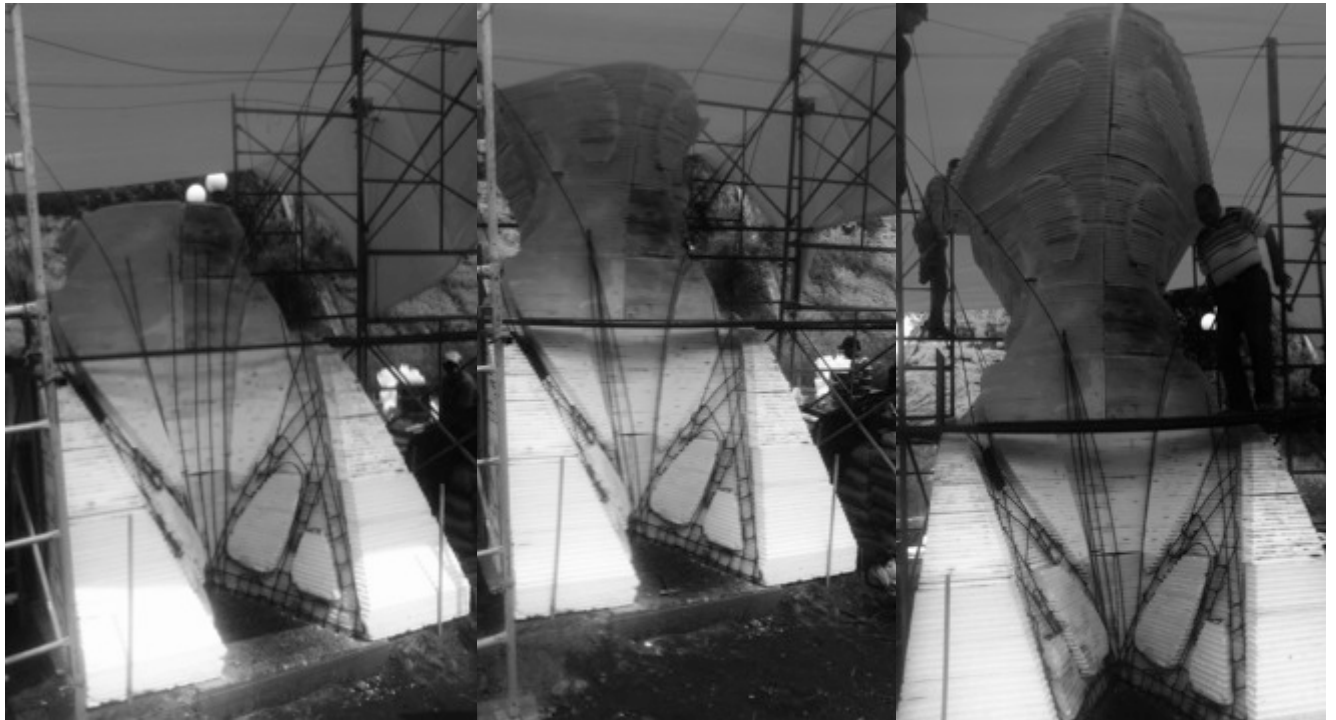
Figure 13: On site assembly of the formwork with scaffolding towers to the sides and placing of the reinforcement bars
