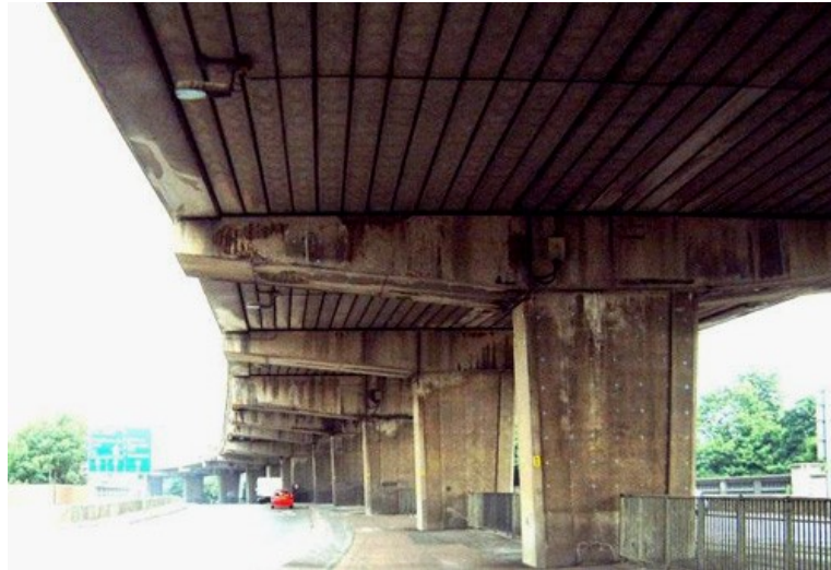
Figure 1.1: Photograph of bridge on the M4 in London, the reinforcement corrosion due to the de-icing salt (Fesi, 2012)
