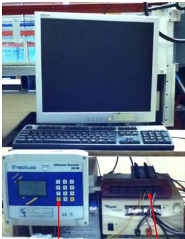
Ultrasonic Flowmeter Control Panel LabJack Datalogger
