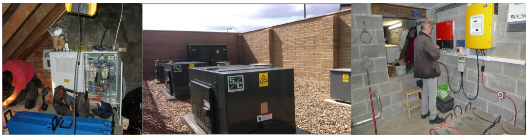
Figure 2: Battery rooms of SoLa Bristol, ZCH and Maes Yr Onn project
