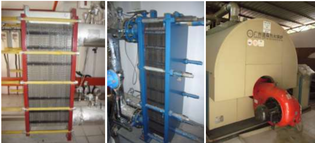
Figure 24 Red plate heat exchanger that heats up the water circulating within the cooling tower circuit (Left) Blue plate heat exchanger that heats up the water circulating within the boiler circuit (Middle) Boiler used to generate heat to heat up water for the experiment (Right)
