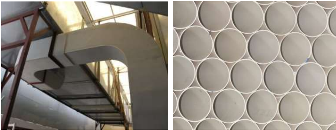
Figure 49 Main air-duct for air circulation (Left) Front view of the circular honeycomb (Right)
