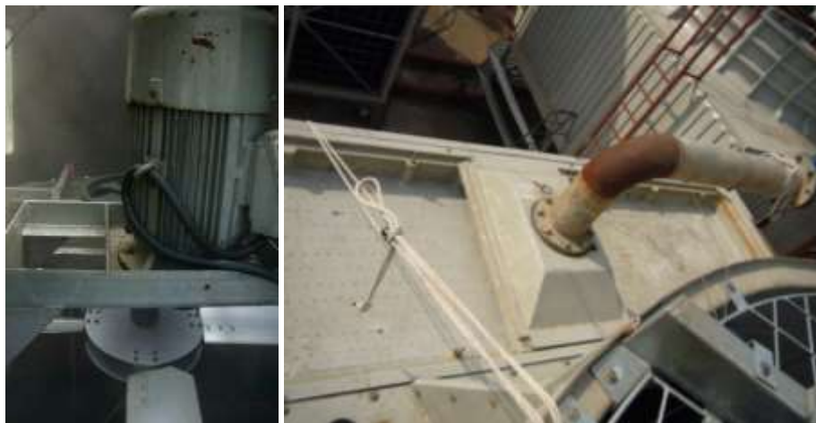
Figure 20 Cooling tower fan and the fan motor at the top of the cooling tower (Left) Installation of the pipe for the cooling tower water inlet (Right)
