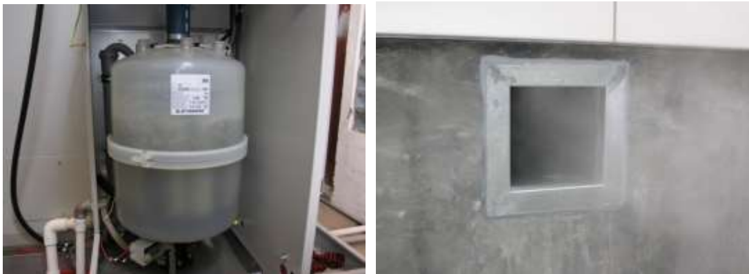
Figure 39 Humidifier that controls the moisture content of the discharge air jet (Left) Opening to discharge humid air while stabilizing discharge air condition (Right)
