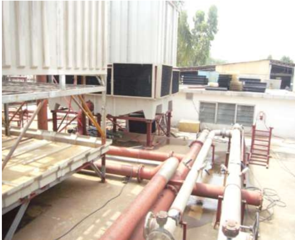
Figure 23 Water piping system used to transport cooling water entering and exiting the cooling tower
