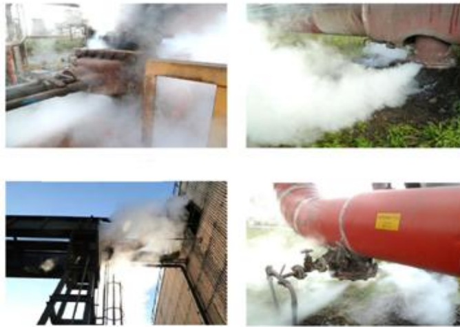
Figure 62 Examples of steam leaks from the distribution circuit
