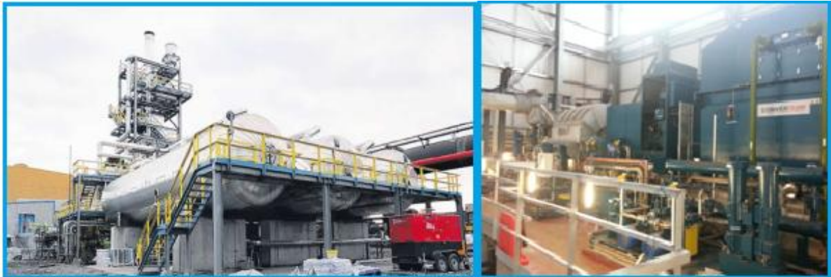
Figure 119: Steam Accumulators, superheater and the new TA in Powerplant
