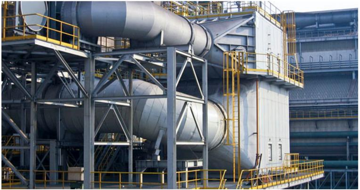
Figure 48 Example Stoves Waste Heat Recovery Unit. (Paul Wurth 2015)
