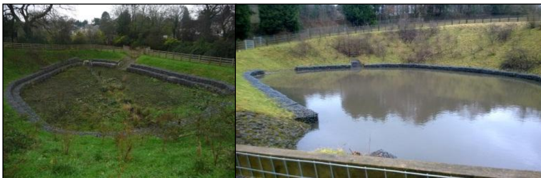
Figure 3-6 - Stormwater pond at Nant y Briwnant, Cardiff: flooded conditions shown on right
