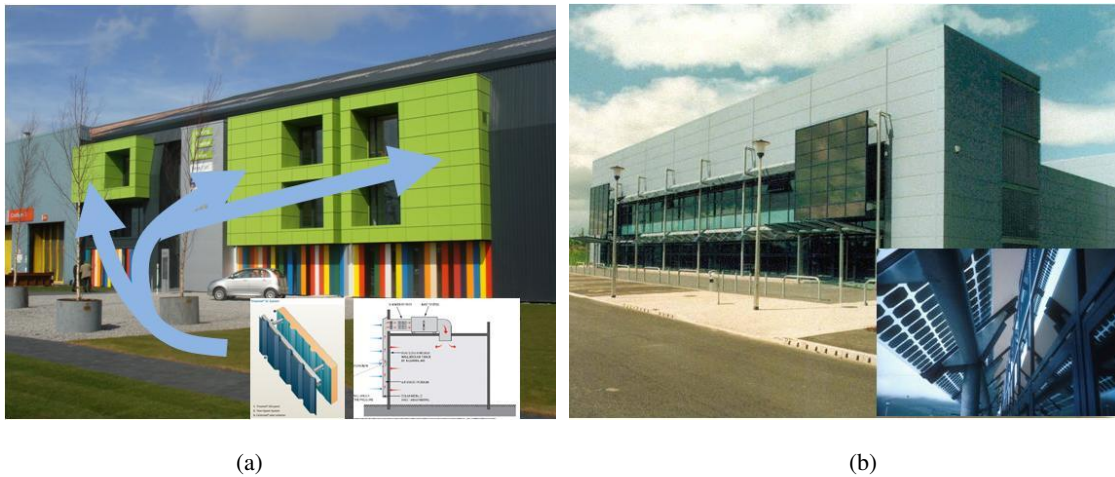
Fig.8 (a) Transpired solar collectors (TSC's) for collecting thermal energy through south facing cladding systems for solar air heating. (b) PV system used as shading device.
