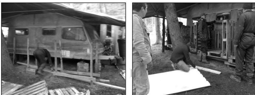
Fig. 6.27 The construction of the log store | Source: left photo: the author; right photo: anon
