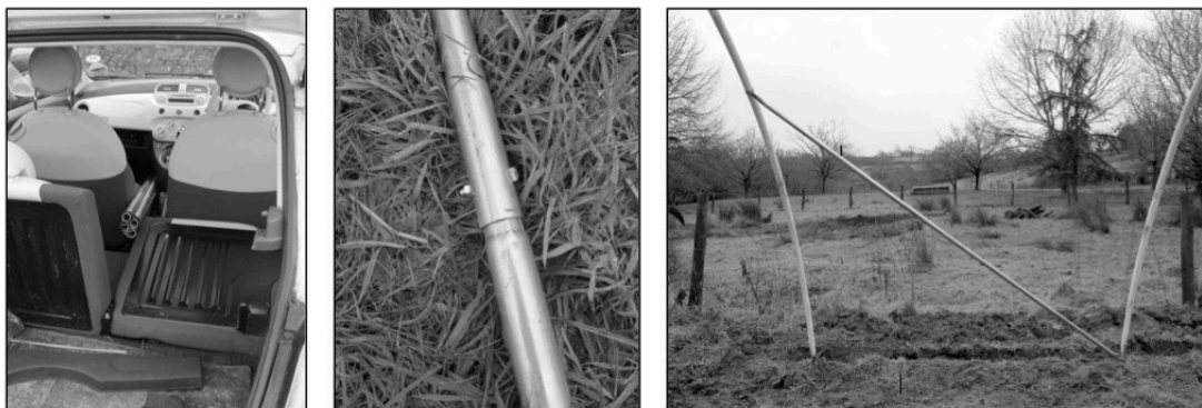
Fig. 6.8 The cross-braces, as transported in a compact car (left); the joint detail between two lengths of tubing (middle); and one of the two completed 3m long cross-braces after installation (right) | Source: the author
