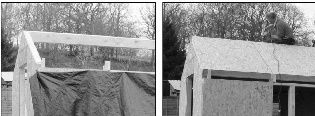
Fig. 6.40 Timber blocks were used to support roof panels after full length profiled timber could not be sourced economically | Source: the author
