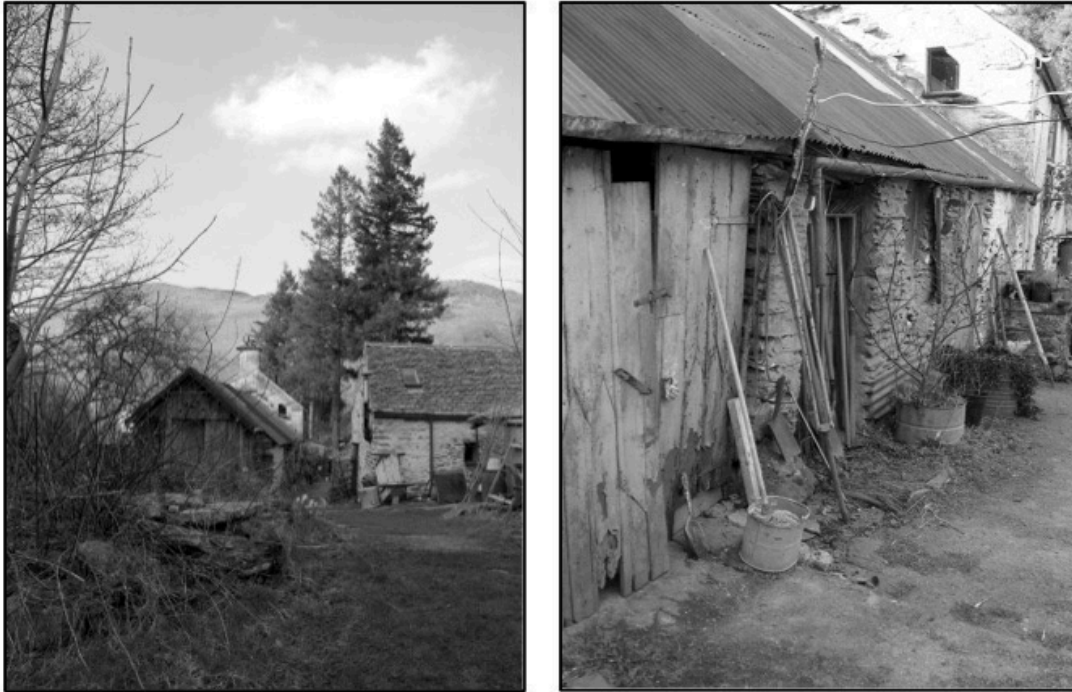
Fig. 4.3 Outbuildings at UC: messy at a detailed scale, picturesque at a large scale | Source: the author
