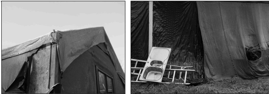
Fig. 7.19 Tarpaulin on the pod beginning to fail (left); and a photograph from the series 'Means of Escape' by Julian McKenny (right)
