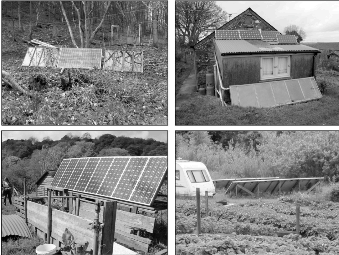
Fig. 4.15 Photovoltaic panels: at BD (top left); at CN (top right); at OD (bottom left); and at GC (bottom right) | Source: the author
