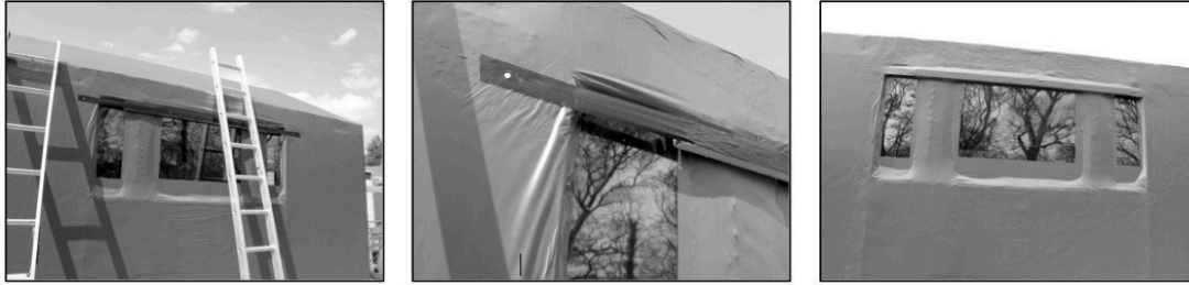
Fig. 6.45 Ad hoc head detail to window to create drip, 21/04/2014 | Source: the author
