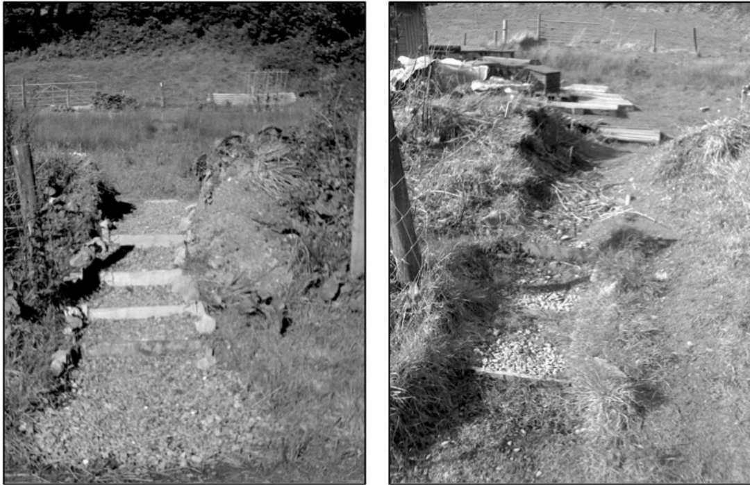
Fig. 6.50 Ad hoc steps to provide access to veg beds at UI, made by my partner and Jon: in September, 2012, soon after their creation (left); and in February 2014 (right)
