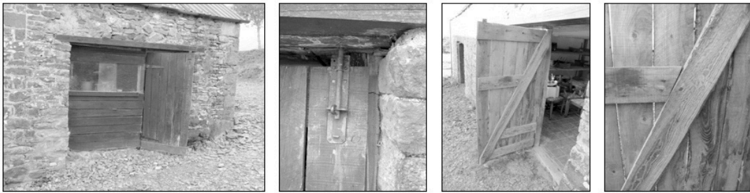
Fig. 6.4 The eastern barn. Rudimentary door and window to storage | Source: the author
