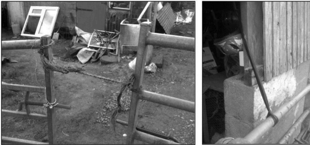
Fig. 6.36 Two different methods for holding gates closed at UI | Source: the author
