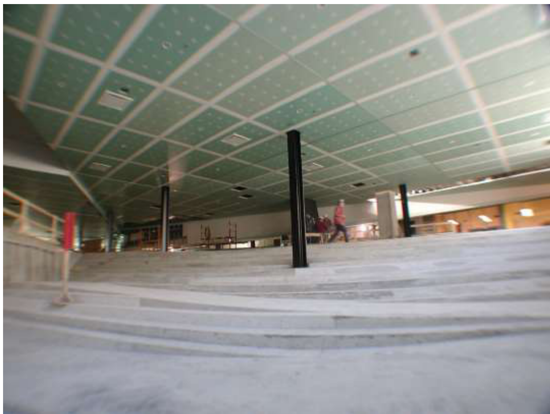
Fig. 10.30 - Image of MTCC ceiling near completion from Mark Schendel to H&R 10 April 2003
