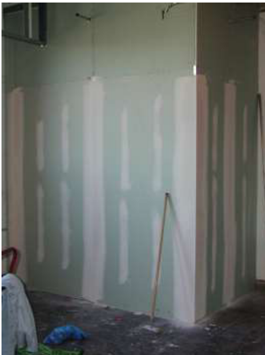
Fig. 10.16- First mock-up of exposed greenboard and spackle at the MTCC, image emailed to OMA NY on 6 March 2002
