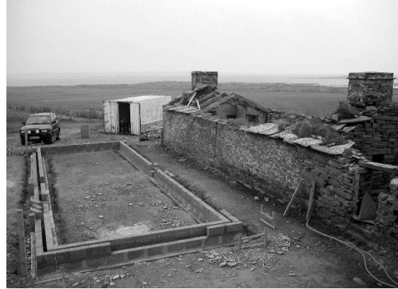
Fig. 2.22 - Concrete block foundation wall of the north addition, Wheelingstone, 2004. All blockwork set out to avoid cutting.
