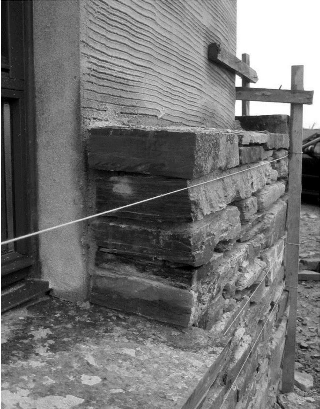
Fig. 2.2 - The wall as constructed: a flagstone, concrete block and timber frame wall at Wheelingstone.
