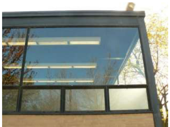
Figure 9.12 - Pressed steel windows at the Commons, IIT (photographed in 2015 by Jan Frohburg).
