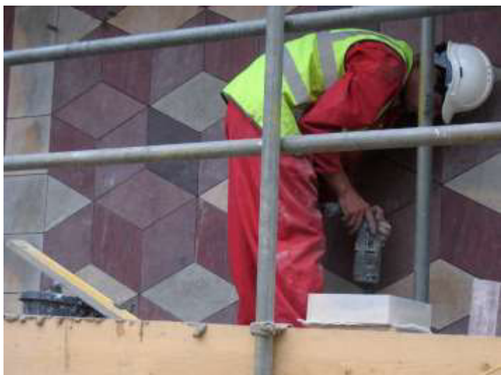
Fig. 8.28 - Construction of the stone cladding, Museum of Childhood, 15 November 2006. Caruso St John Architects.
