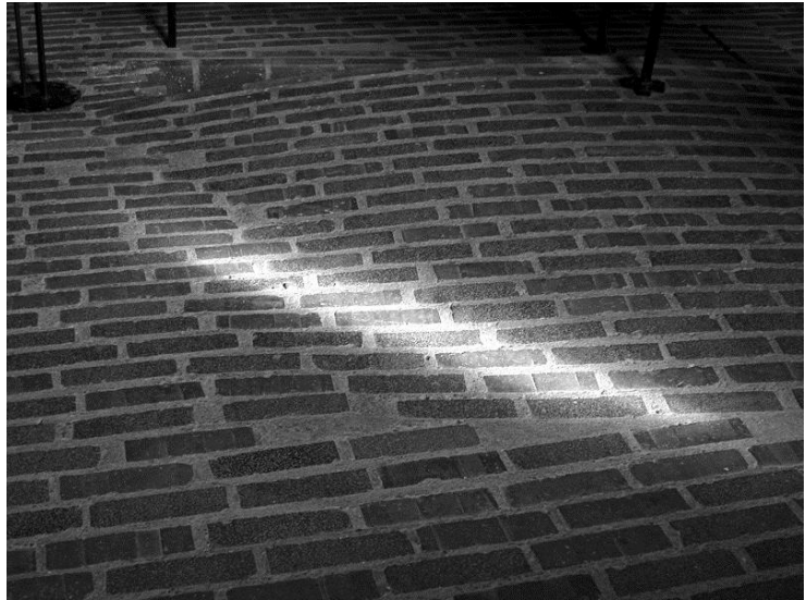
Fig. 3.6 - Mortar joints at St Peter's, interior floor.
