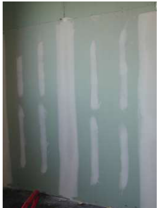
Fig. 10.17- First mock-up of exposed greenboard and spackle at the MTCC, detail emailed to OMA NY on 6 March 2002
