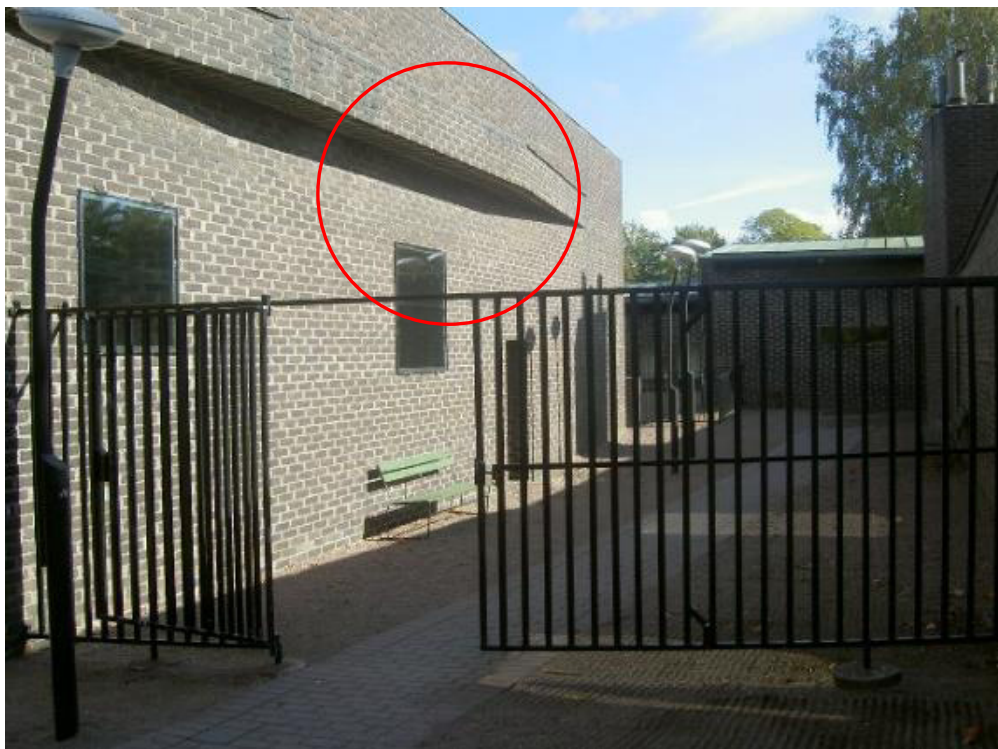
Fig. 3.16 - Deviation from a stringently applied rule: a cut brick, facade, observed and photographed by Simon Unwin.
