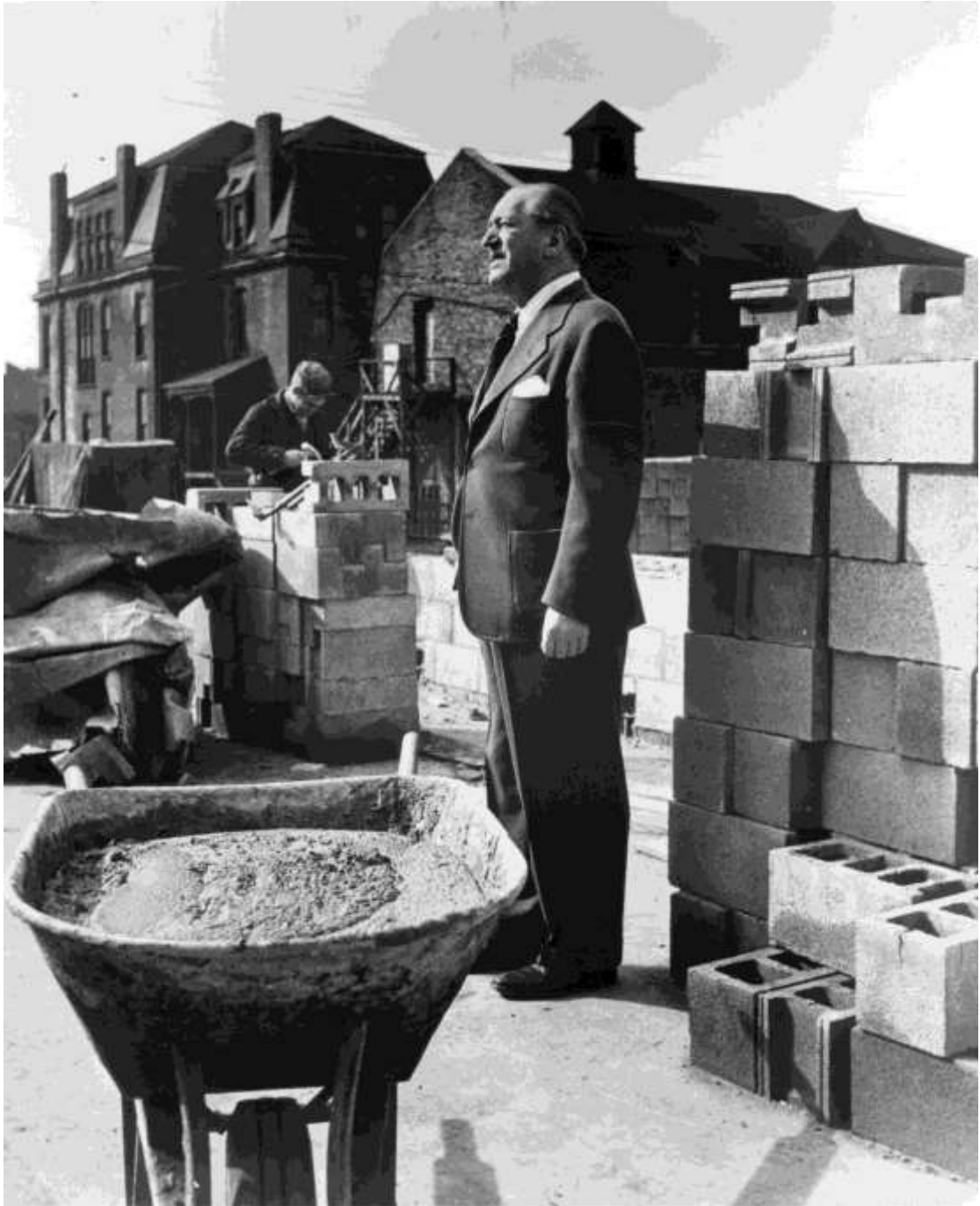
Fig. 9.2 - Mies van der Rohe on construction site at IIT. Main Building is in the background to the south-west, suggesting that this may have been the construction of Navy (Alumni), Perlstein and Wishnick Halls in 1946-1947. University Archives and Special Collections, Illinois Institute of Technology, Galvin Library: 1998.033 Biographical file.
