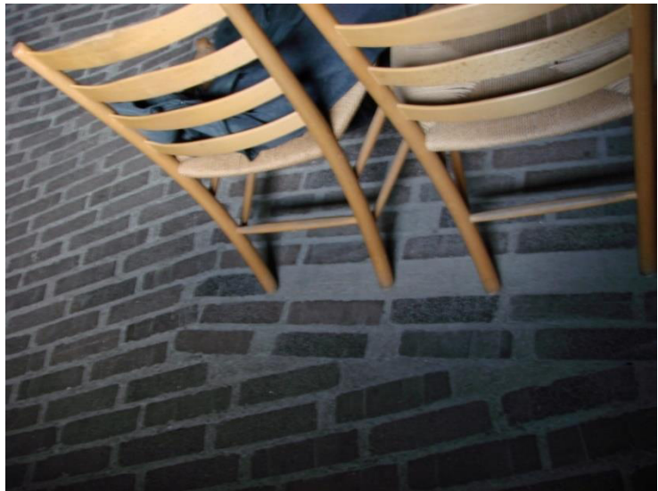
Fig. 3.7 - Mortar joints at St Peter's, interior floor.
