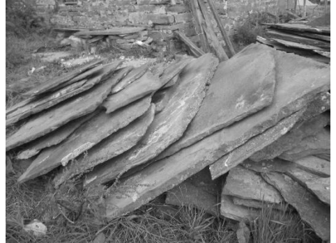
Fig. 2.9 - Collapsed flagstone roof slabs at Wheelingstone.
