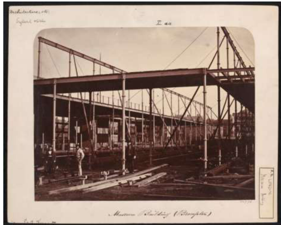
Fig. 7.6 - Exterior view of the South Kensington Museum (the 'Brompton Boilers') under construction looking south east, 1856. Lance Corporal B.L. Spackman, photographer. Commissioned by Department of Science and Art of the Committee of Council on Education. © Victoria and Albert Museum: No.34976.
