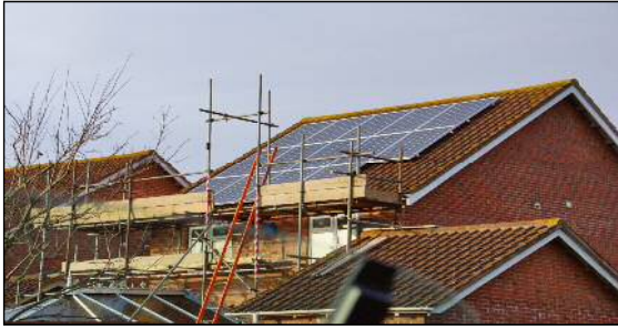
Solar Panels on Roof
