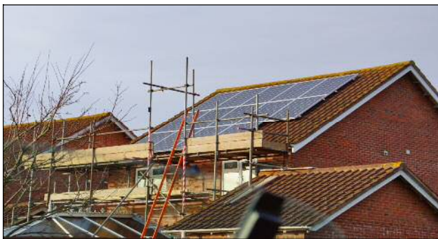
Figure 6: Solar Panels on a Roof 44
