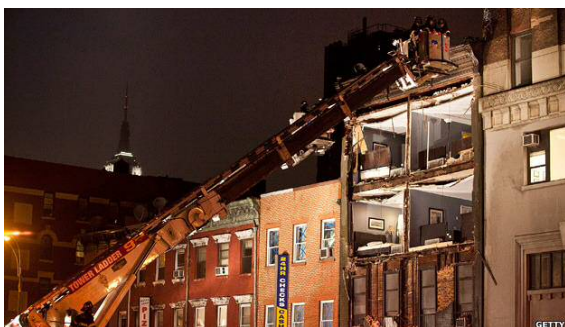
Façade Blown Apart By High Winds
